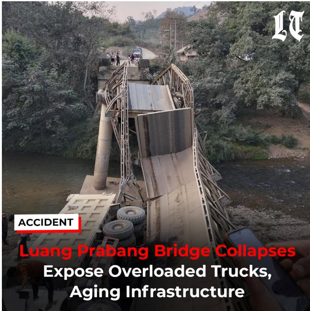
Figure 6. Not just Highway 9 , Bridge collapse in Luang Prabang attributed to overloading, February 09, 2026. Laotian Times.
