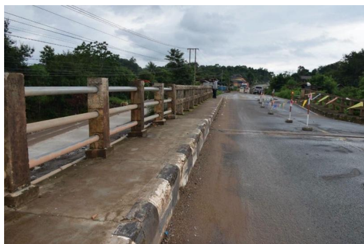
Figure 2. The Huaypaxuan bridge on National Road No. 9 in Xepon district, Savannakhet province, is closed for three months after serious faults were found in the road surface.
